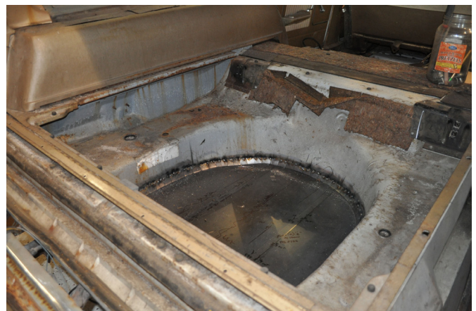
As one of their first welding projects, Berger and Varcoe restored the floor of the trunk.
